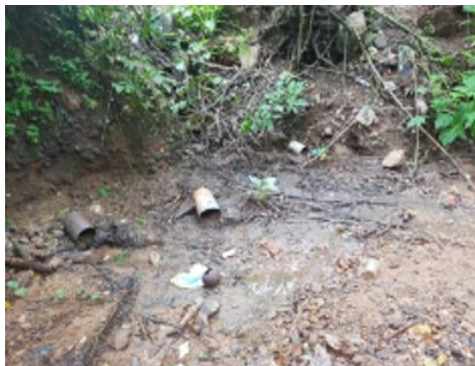
Figure 2. Pipe that pours waste water into the river.
