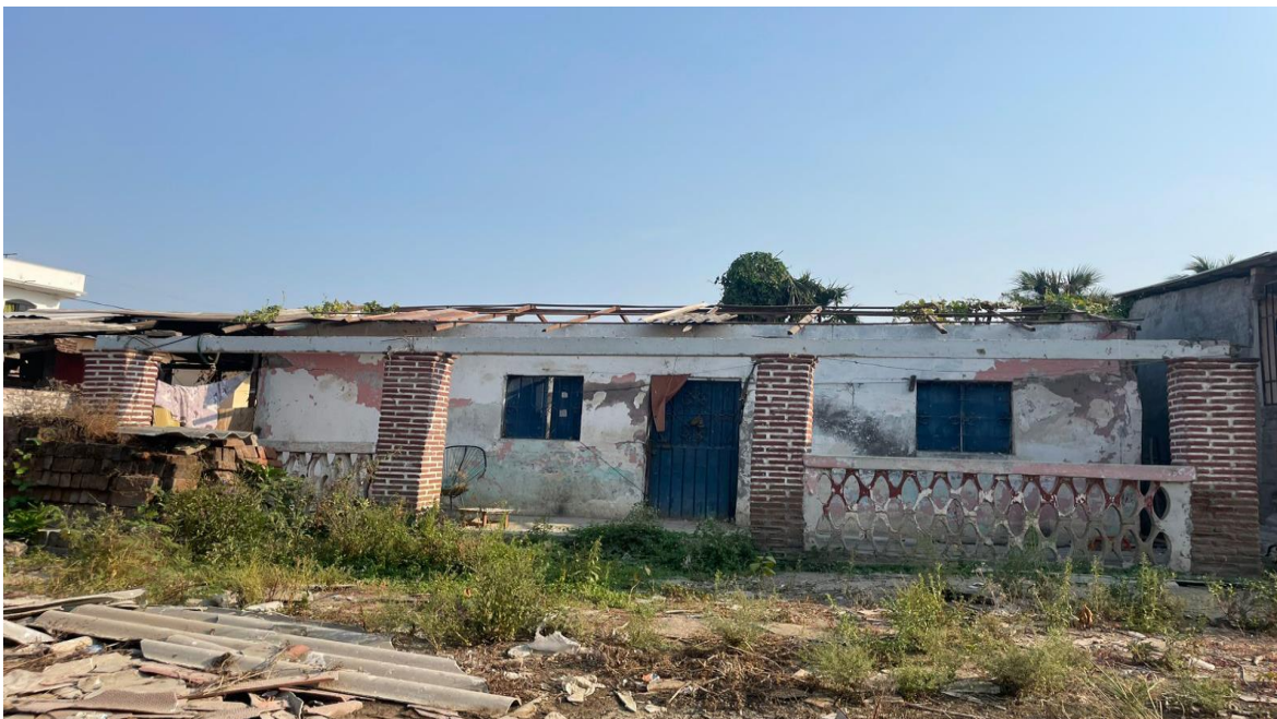
Figure 4. Loss of roofs from homes due to Hurricane Otis.
